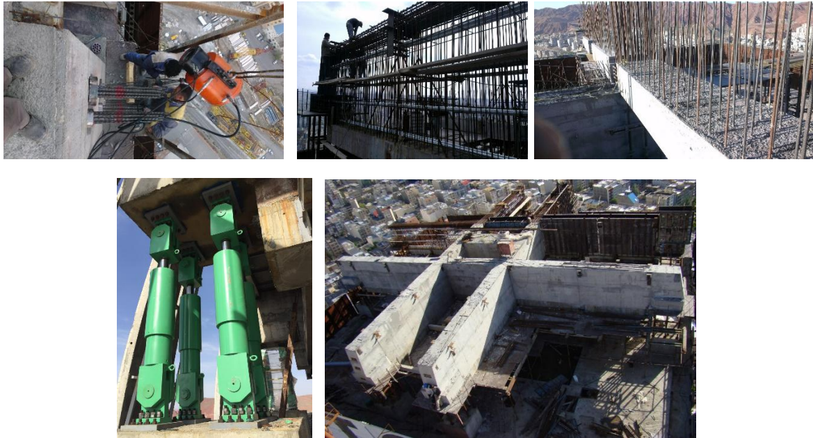
Figure 8- Photos of super beams construction and viscous dampers installation in WTC Tabriz building
